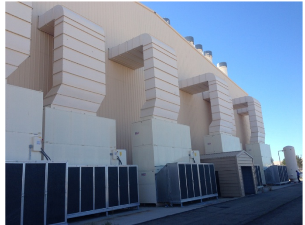
Figure 1: Good duct install
