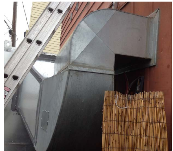
Figure 2: Poor duct install
